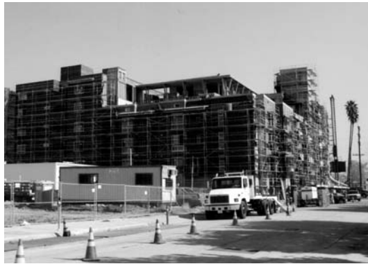
Design guidelines are needed to improve the way buildings address the public realm, avoiding residential buildings such as these that loom over the street with no setbacks or open areas.
