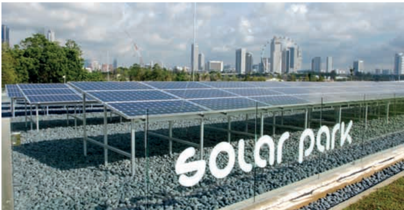
The solar park in Marina Bay is the largest field of solar panels in Singapore, generating 50 per cent of the daytime electricity needs of the Marina Barrage facility. Photo courtesy of PUB, Singapore's national water agency.
